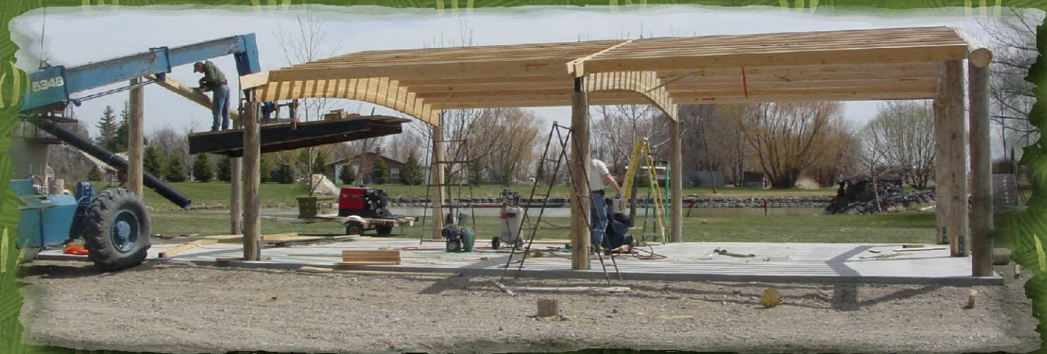
The large trusses made it possible to span the roof without poles in the middle
